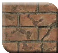
FIRE CRACKED BRICK
